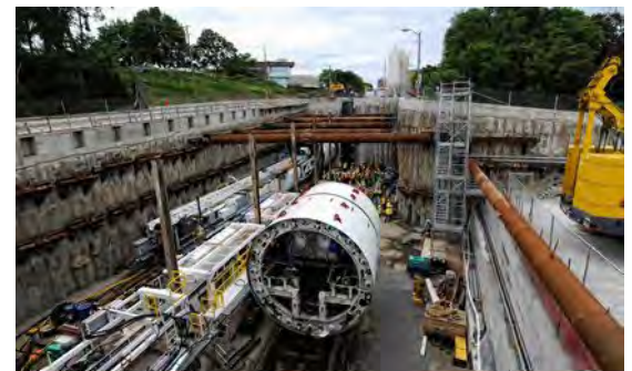
Site at Black Creek Drive where the tunnel boring machines begin tunnelling
